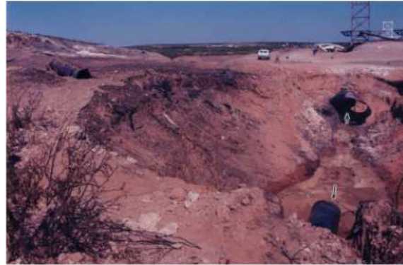
Photo 5: Carlsbad Rupture Crater (Courtesy of NTSB)
